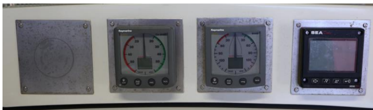
Wind instruments located above the companionway hatch
